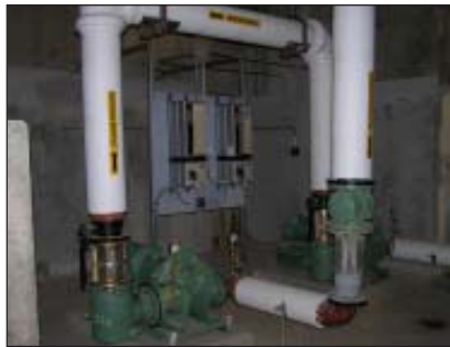
VFD Pumping Systems
