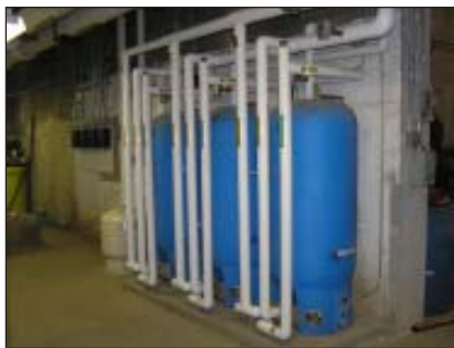
Hot Water Generators
