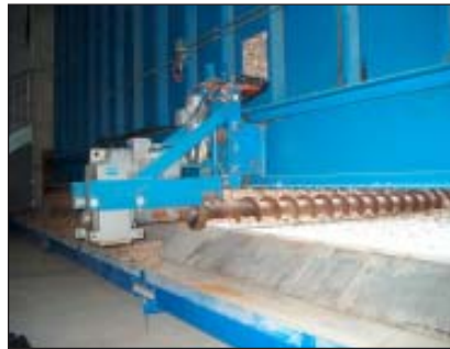
Wood Chip Boiler System
